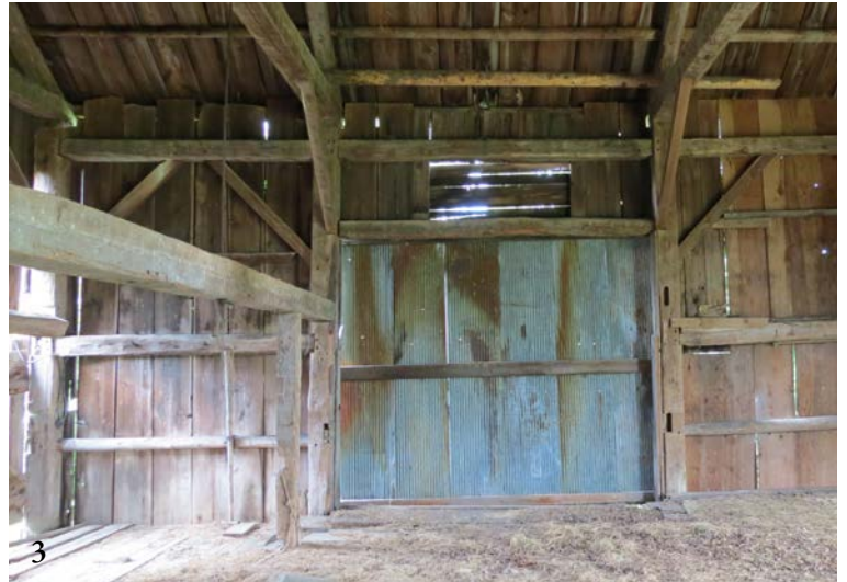
3 A Newbury, VT, threshing barn probably built for the Fulton family circa 1830. An uncommon, resilient frame design using segmented and flying plates, and common purlin roof framing.
